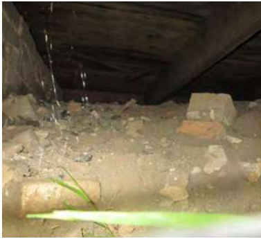
Underside of rear kitchen addition floor, with broken floorboards visible. (ERA, 2017)
