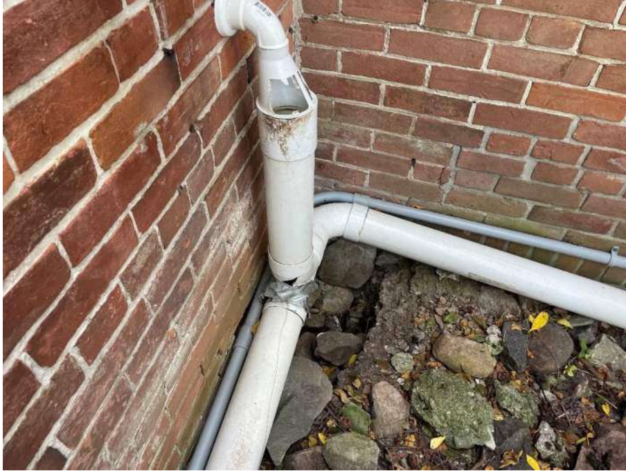
Photo 1: Damaged downspout hard piping.
