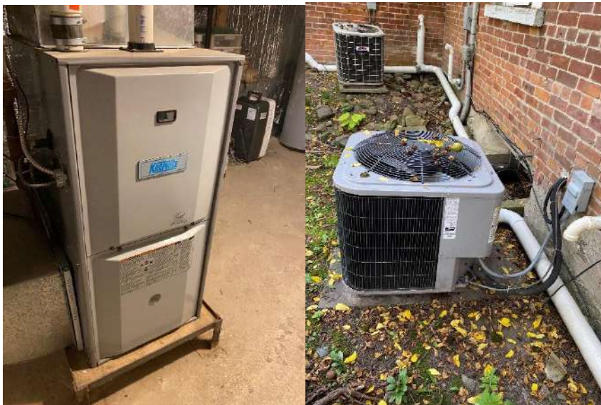
West Mechanical Room Furnace and associated outdoor air conditioning unit.
