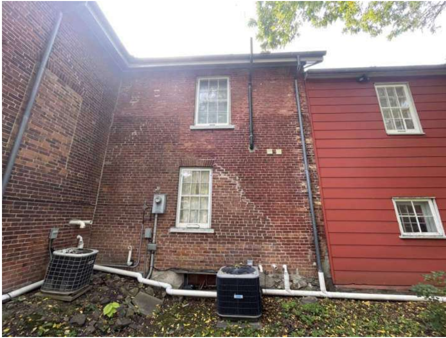
Photo 3: Cracking double brick wall
