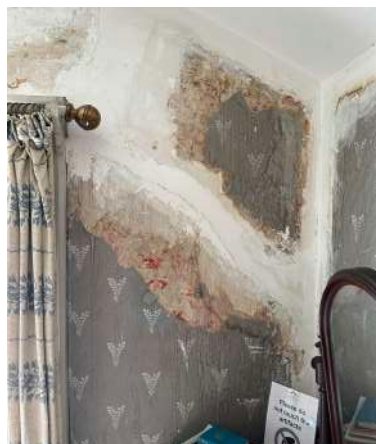
Deteriorations of wall paper with emergency plaster repairs in bed rooms on second floor. (ERA, 2023)
