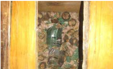
Hole to be repaired at second floor washroom. (ERA, 2017).
