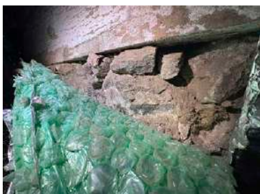
Uncovered, deteriorated fieldstone foundation under waterproofing in basement.
