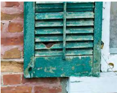
Wood shutter has been chewed, allowing access to a hole in the masonry. (Hillary House National Historic Site, 2017).
