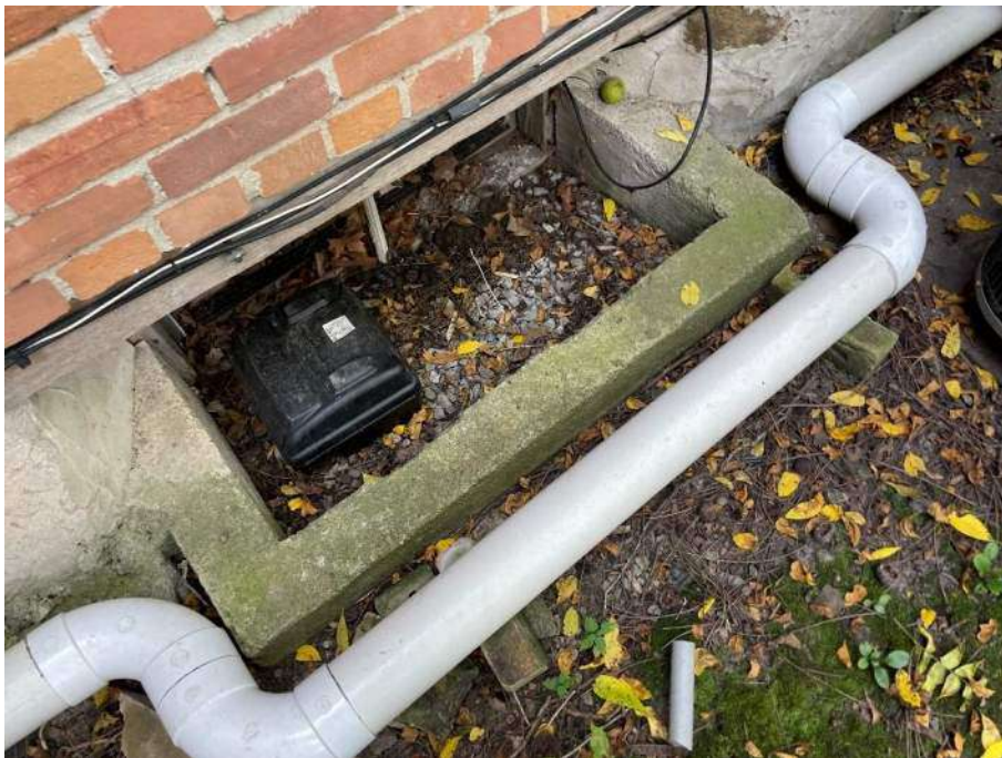
Photo 4: Improper water management at window well
