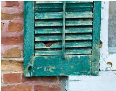
Any animals should be removed and the shutter and masonry repaired. (Hillary House National Historic Site, 2017).
