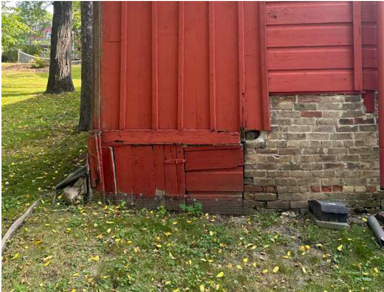
Animal Ingress routes through the summer kitchen north-west corner which have been partially addressed with chicken wire, and traps. Note, significant amounts of skat present in outhouse. (ERA, 2023)
