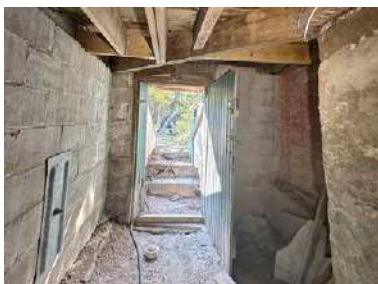
One of 2 capped off drain pipes under south verandah crawl space.
