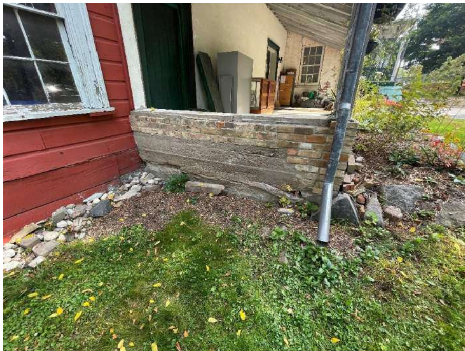
Photo 8: Phase 3 porch slab on grade without proper frost protection
