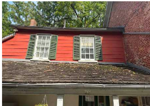
Moss seen on 1888 addition verandah cedar roof.
