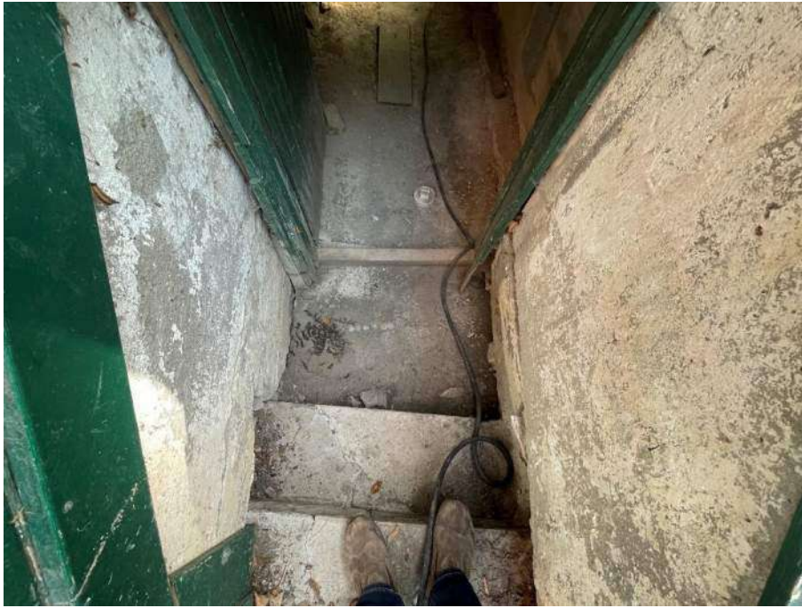
Photo 5: Missing drain at base of walk-up stairs
