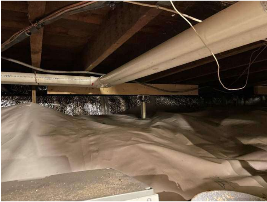
Photo 9: Over spanned floors in basement (Phase 1) – temporary supports added
