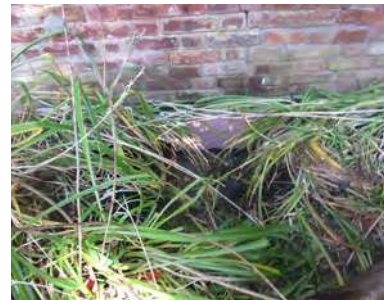
Depression in ground by site of former coal chute at south elevation. (ERA, 2017).
