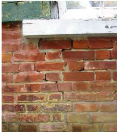
Left: South elevation of 1869 Addition. Right: Structural cracking beneath 1st story window at south elevation of 1869 addition. (ERA, 2017)
