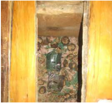
Cavity in historic washroom floor showing evidence of animal infestation. (ERA, 2017)
