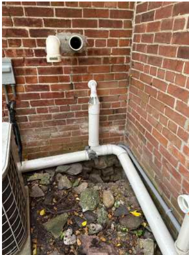
Rupture at PVC pipe with wash-out of backfill at foundation.
