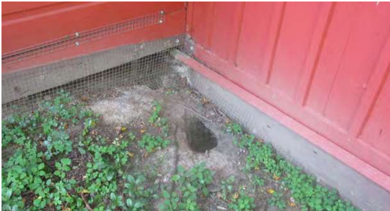
Evidence of burrowing animals under floor structure of rear kitchen addition at north elevation. (ERA, 2017)
