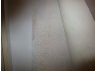
Delaminating wall paper at second floor bedroom (now gallery). (ERA, 2017).
