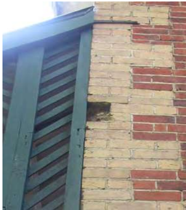
Left: West facing elevation of main house. Right: Missing brick units at this elevation. (ERA, 2017)
