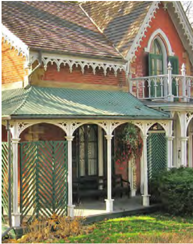
Portion of east veranda where firmness issues are present in the floor. (Wikimedia Commons).
