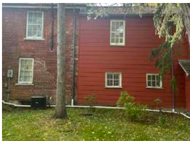
PVC rain water pipe collecting water from 5 rainwater leaders.
