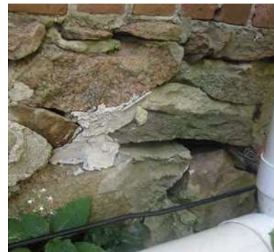
Detail of deteriorating foundation at north elevation of 1869 addition. (ERA, 2017).
