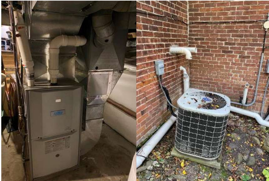
East Mechanical Room Furnace and associated outdoor air conditioning unit.
