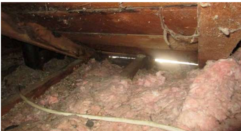
Area of potential animal entry at eaves of 1869 addition roof, showing disturbed batt insulation at assumed entry point. (ERA, 2017)
