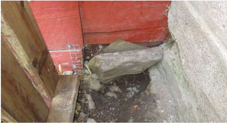
Potential point of animal entry at south portion of rear kitchen addition. (ERA, 2017)
