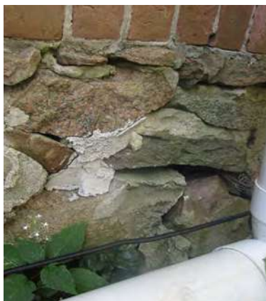
Left: North elevation of 1869 addition Right: Detail of deteriorating foundation at north elevation. (ERA, 2017)
