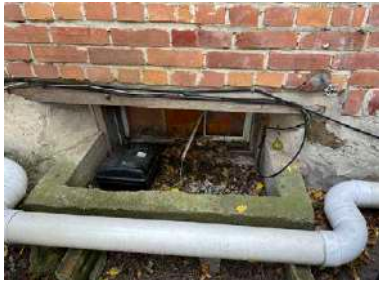
1869 addition north elevation window well with broken window.
