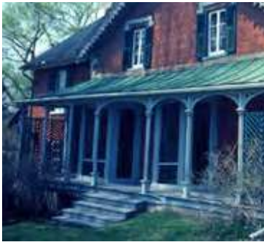
Portion of north veranda where firmness issues are present (Parks Canada).
