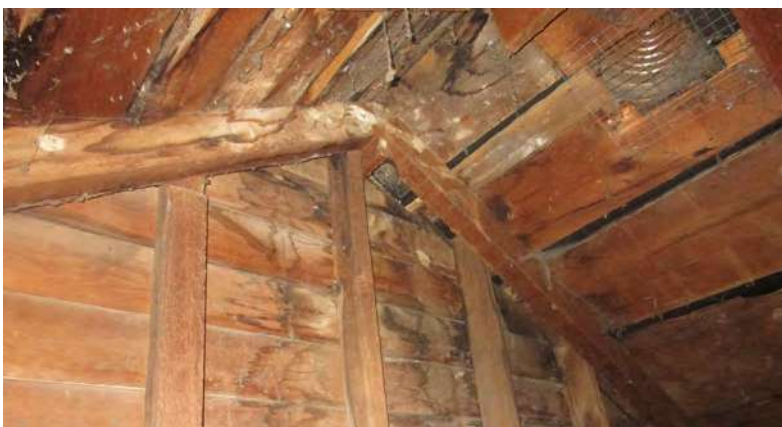
Area of water penetration at west gable of western attic. (ERA, 2017)
