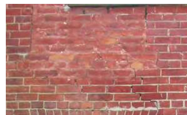
Base of infilled door at north elevation, with step crack visible. (ERA, 2017).
