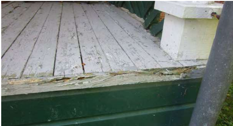
Deteriorating woodwork at Veranda edge. (ERA, 2017)
