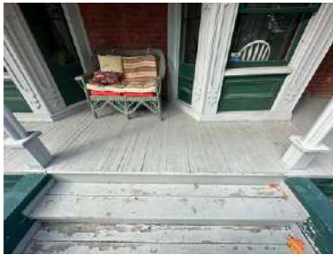
Deficient paint work at exterior west veranda stairs.
