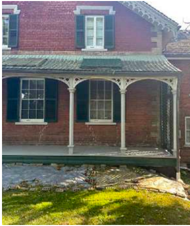
North Verandah missing stairs to tennis court.
