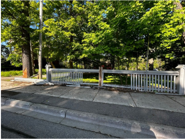
Damage to Fence, May 2024
